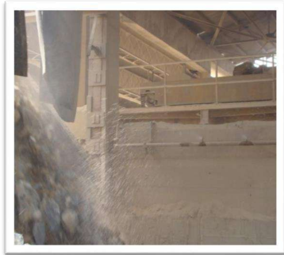
Water spraying System in Crusher Hopper
